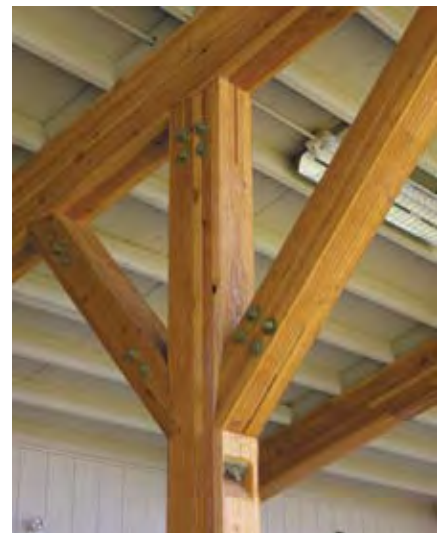
Equilibrium Consulting re-engineered the driving range project, using notches and hidden connectors to save money. The strategy also resulted in a clean, uncluttered design.
